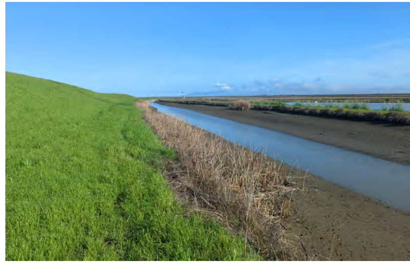
Representative photo of levee hillslope and ditch of Site A and Site B, facing northeast. Photo taken February 22, 2024.
