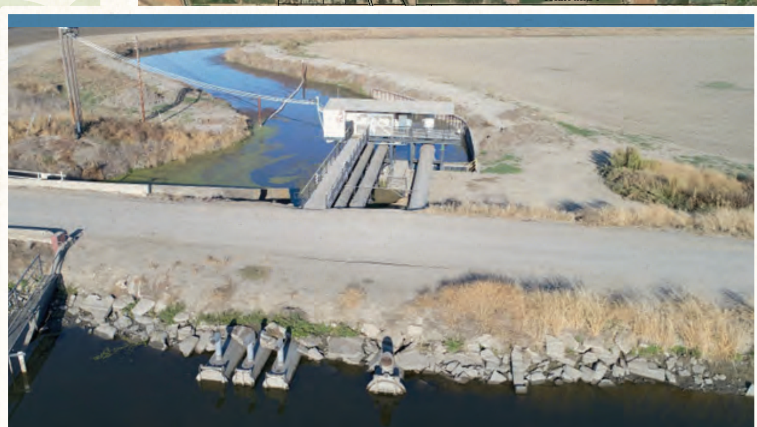
SYCAMORE Drain water can be reintroduced to the District's delivery system through four pumps with a maximum capacity of 270 cfs.
