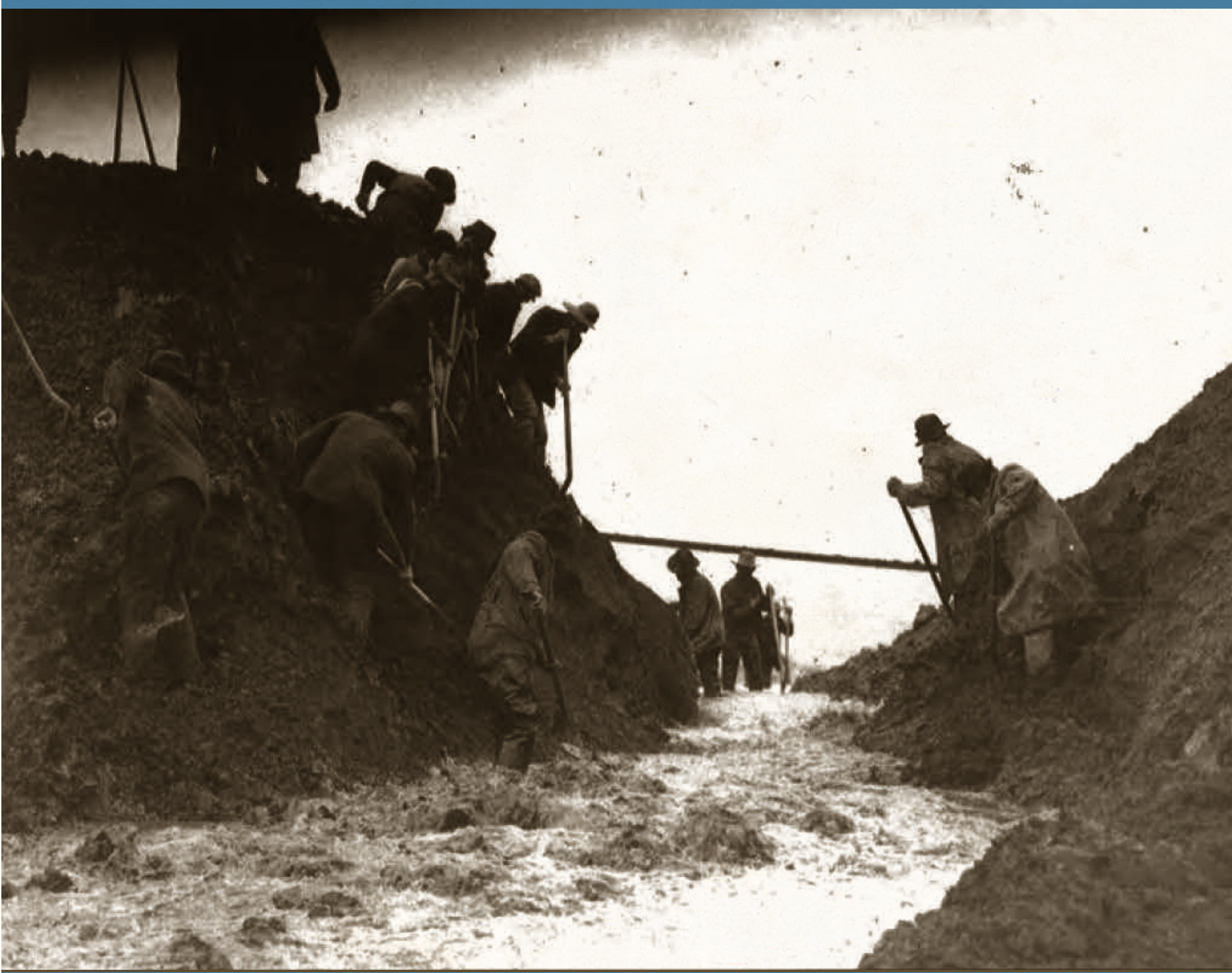
DREDGE "JIMENO" ENLARGING OPENING THROUGH DAM AT HEAD OF RIDGE CUT. 4:30PM, FEBRUARY 22, 1915
